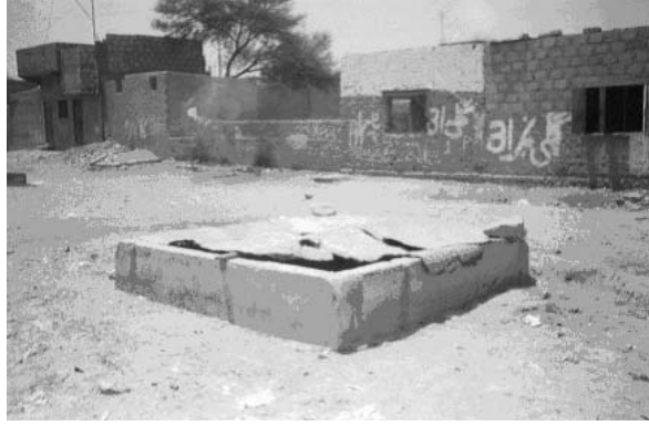
Photograph 5.21. An awami tank at Christian Mohalla, Ghaziabad, Sector 1½, Orangi Town. The tank is covered with broken sheets and gets polluted with dust and other impurities. The physical surroundings are a hazardous situation.
