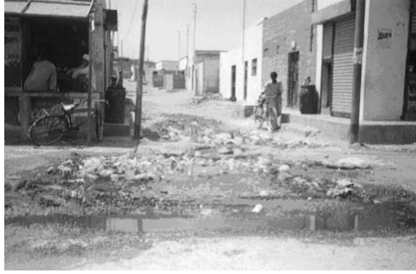
Photograph 5.18. View of a lane in Ghaziabad. Stagnant water often seeps through the underground tank causing contamination and health hazards
