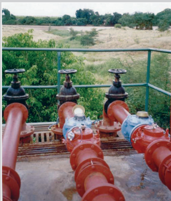
Photograph 7.1. Commercial tube-well and infiltration scheme using submersible pumps.
