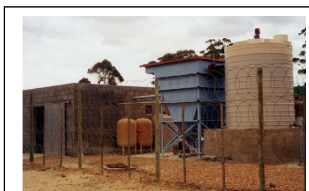
Figure 2. The conventional water treatment plant
