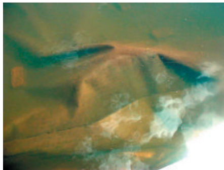
Figure 3. Negative pressures lifting SSF fabric material in Tulbagh
