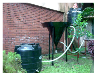
Photograph 6. 100 L/h prototype system temporarily installed at BUET for testing
