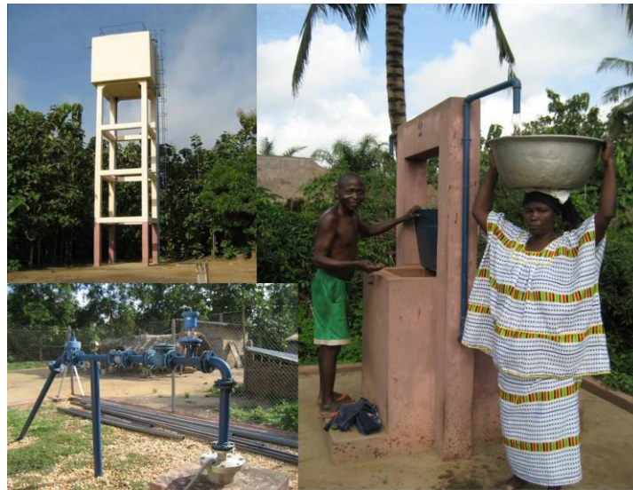
Photograph 1. Components of a piped network. Clockwise from bottom left: borehole; water tower; and standpost with water seller and user
