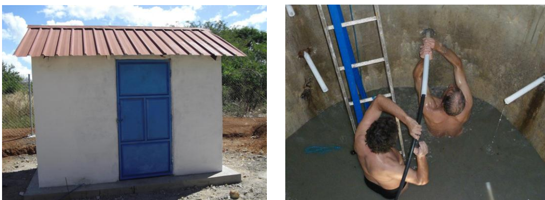
Figure 3. As part of the “permanentization” proper pump houses were built (left). To increase extraction of water while carefully using the top layer of the limited fresh groundwater, horizontal filter pipes were flushed into the sandy soil up to 6 meters out from the central large diameter well (right).
