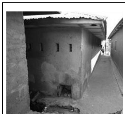
Figure 2. Closed down bucket toilets in the compound house of Figure 1.
