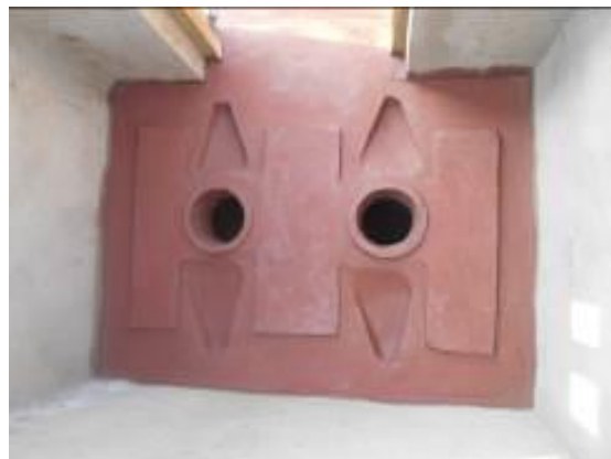
Photograph 2. Locally modified toilet
