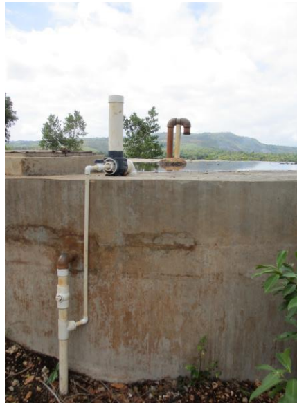
Photograph 1. WEDC - Chlorinator installed on a reservoir in Southeast, Haiti
