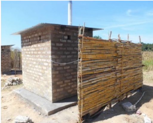
Photograph 6. Low-cost school toilet
