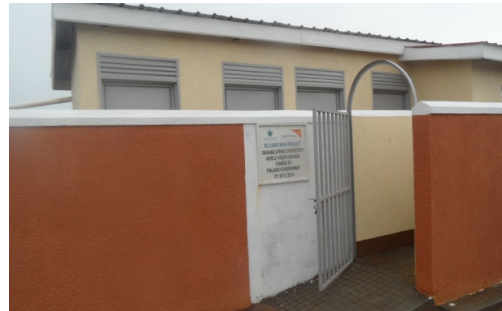
Photograph 1b. Toilet constructed in a school within the refugee camp
