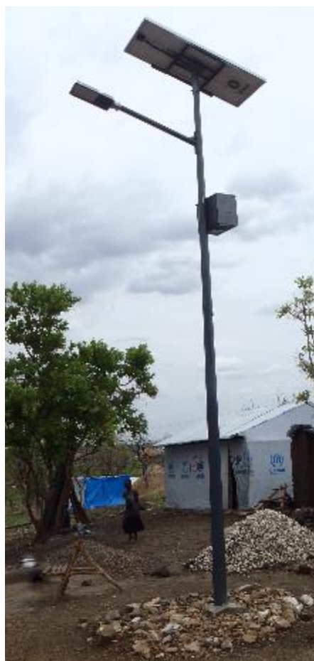
Photograph 1. An installed lamppost
