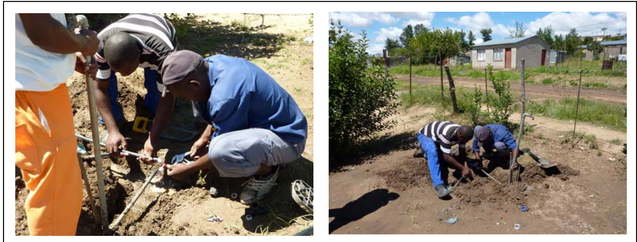
Figure 2: Leak repairs in Ficksburg Township
