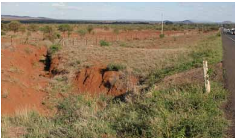
Figure 64. Along the road to Nairobi (from Mombasa), Kenya. The government constructed cross-cutting drainage ditches under this road to drain it. This farmer uses these structures by digging a ditch and leading the drainage water in to his farm. As this ditch is unprotected it could turn into a deep gully after a rainy season flushing away valuable top soil. (photo: MetaMeta).
