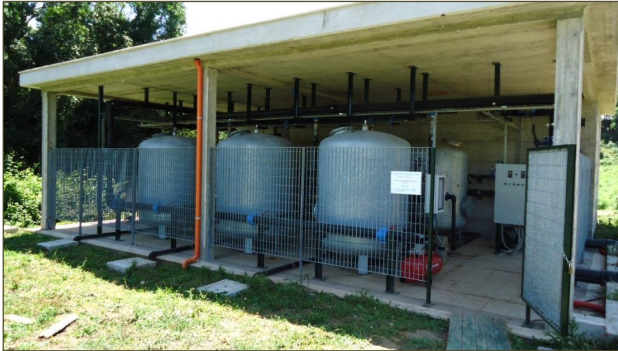
Figure 5.6 The arsenic removal plant (Photographed by the author)
