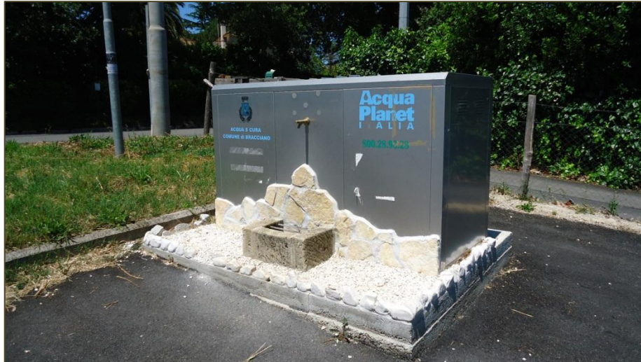
Figure 5.5 Public standpost on Via della Macchia (Photographed by the author)
